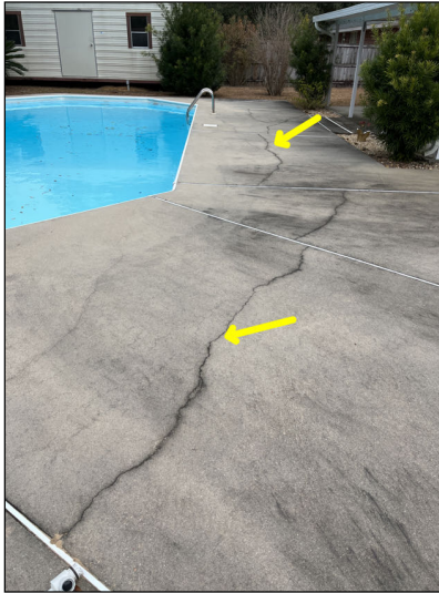
Cracks in concrete decking noted. Recommend repair
