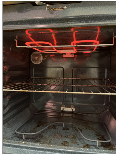
All heating elements operated when tested.
