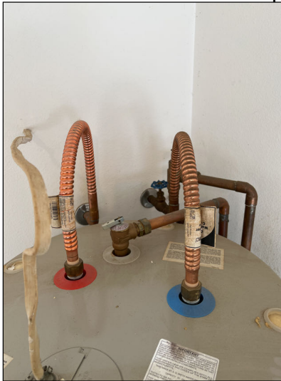
No deficiencies observed at the visible portions of the supply piping.
