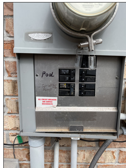
No major system safety or function concerns noted at time of inspection at main panel box.
