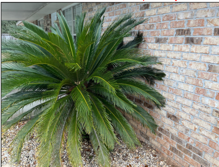
Prune or remove any plants that are in contact or proximity to home to eliminate pathways of wood destroying insects.
