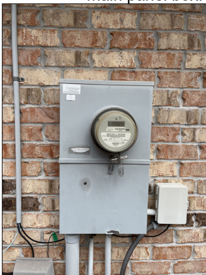
No major system safety or function concerns noted at time of inspection at main panel box.
