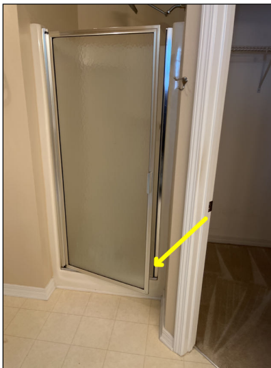
Shower door is difficult to close. Recommend adjustment.
