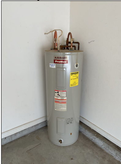
Tank is in satisfactory condition -- no concerns.
