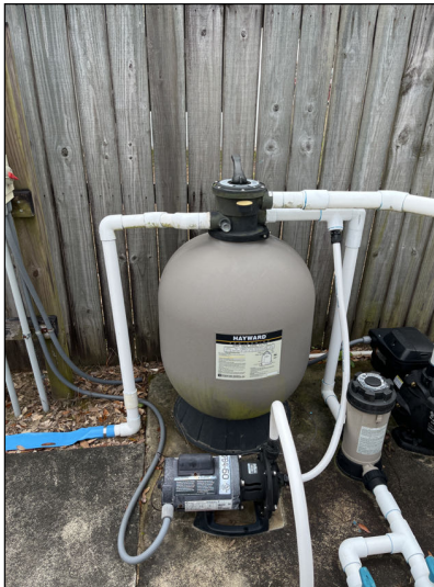
Sand filter noted.
