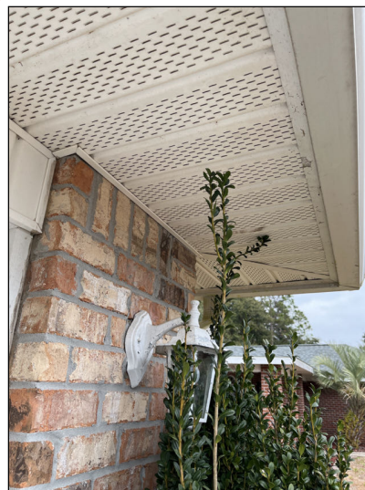
Prune or remove any plants that are in contact or proximity to home to eliminate pathways of wood destroying insects.
