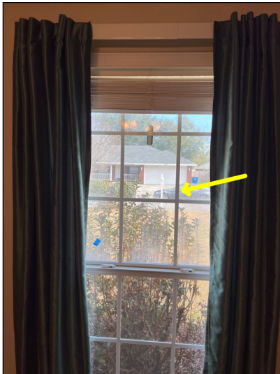
Fog/condensation observed in thermopane windows. This is an indication of a failed seal. Recommend review for repair or replacement as necessary.
