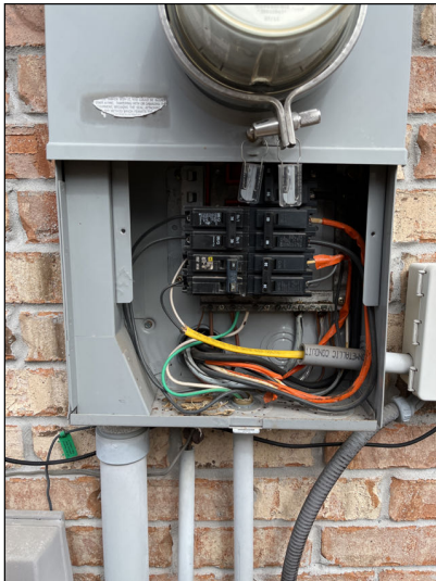
No major system safety or function concerns noted at time of inspection at main panel box.
