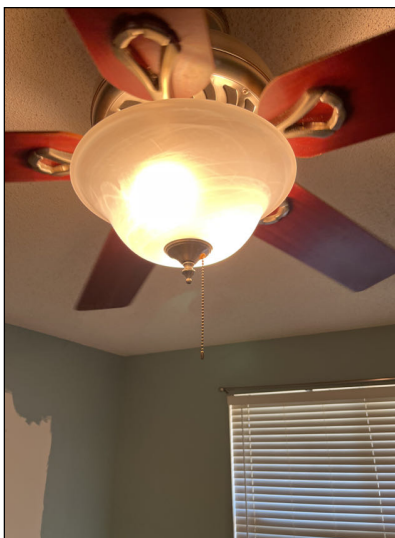
The ceiling fan pull chains did not operate when tested.
