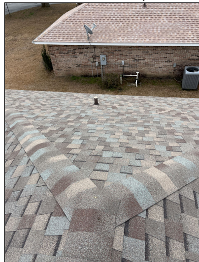
No major system safety or function concerns noted at time of inspection.
