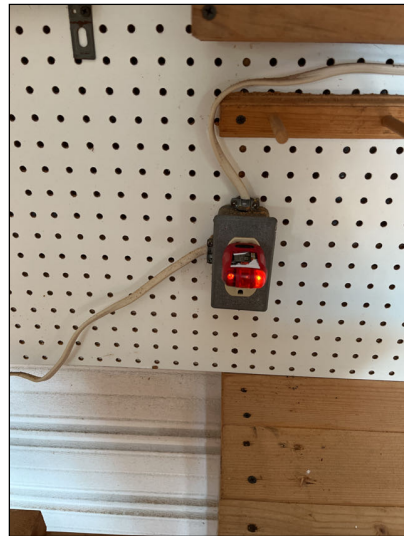
Hot/Ground reversed on all outlets, recommend repair
