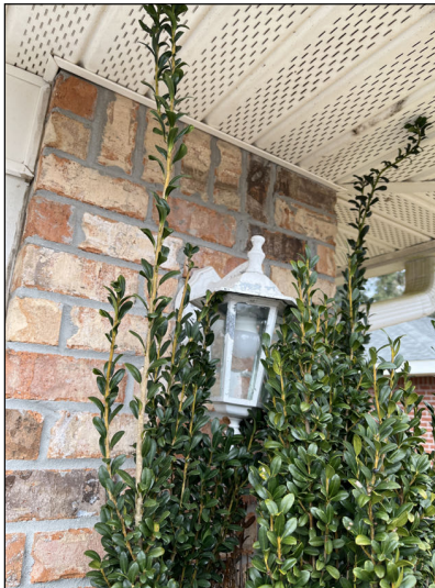
Exterior light out, recommend replacing bulbs then testing.
