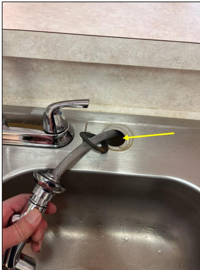
Spray wand needs re-securing.
