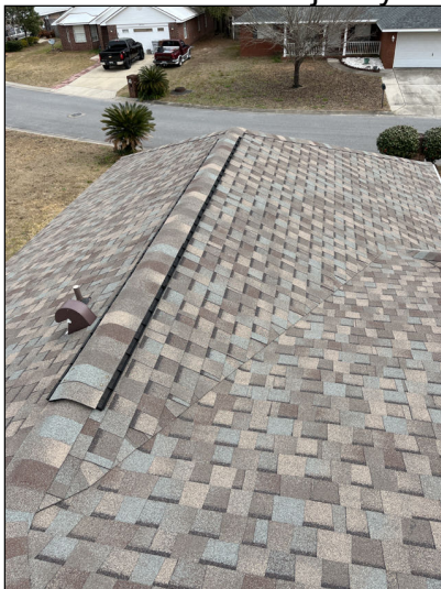
No major system safety or function concerns noted at time of inspection.
