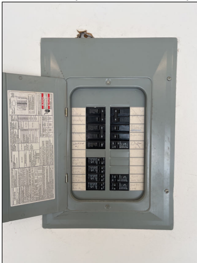
No major system safety or function concerns noted at time of inspection at main panel box.
