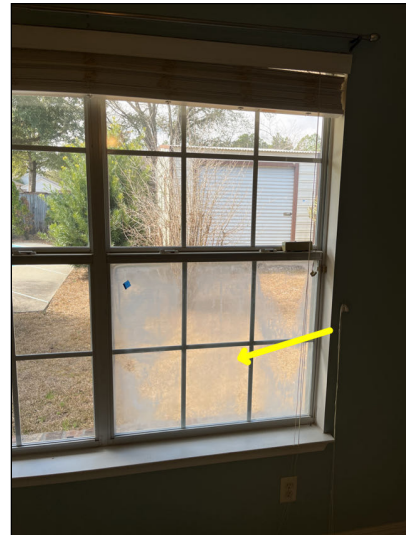
Fog/condensation observed in thermopane windows. This is an indication of a failed seal. Recommend review for repair or replacement as necessary.
