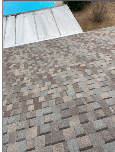
No major system safety or function concerns noted at time of inspection.
