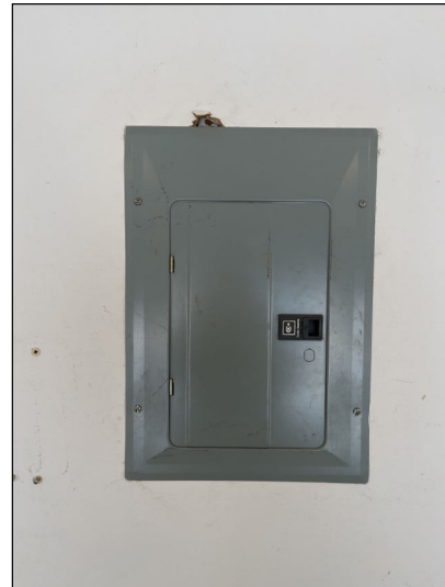
No major system safety or function concerns noted at time of inspection at main panel box.
