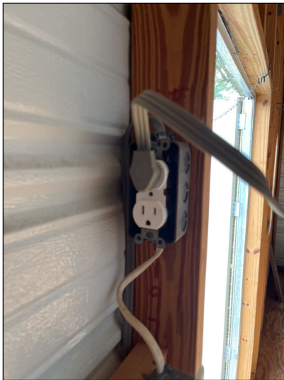
Outlet covers missing
